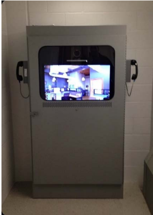
Figure 1. Correctional Video Unit with the Privacy Phone
